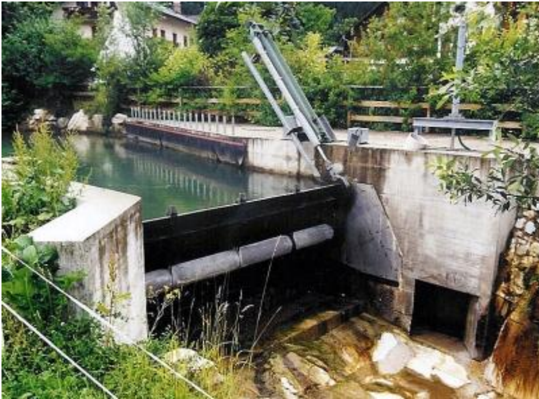
Figure 4.5. Example of a hydraulic tilt gate used to simulate overshoot flow (Photo Courtesy of Waterpower Engineering, UK).
