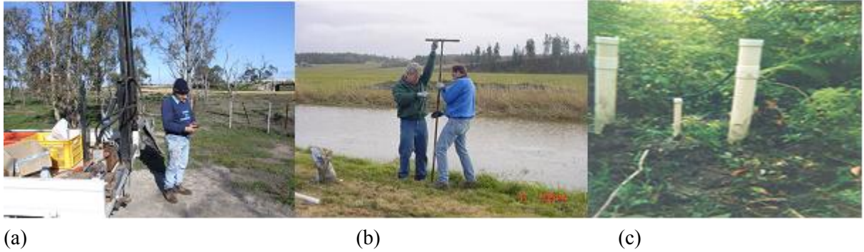
Figure 7: Piezometers are used for monitoring the watertable: (a) drilling bores, (b) installation, and (c) a set of piezometers
