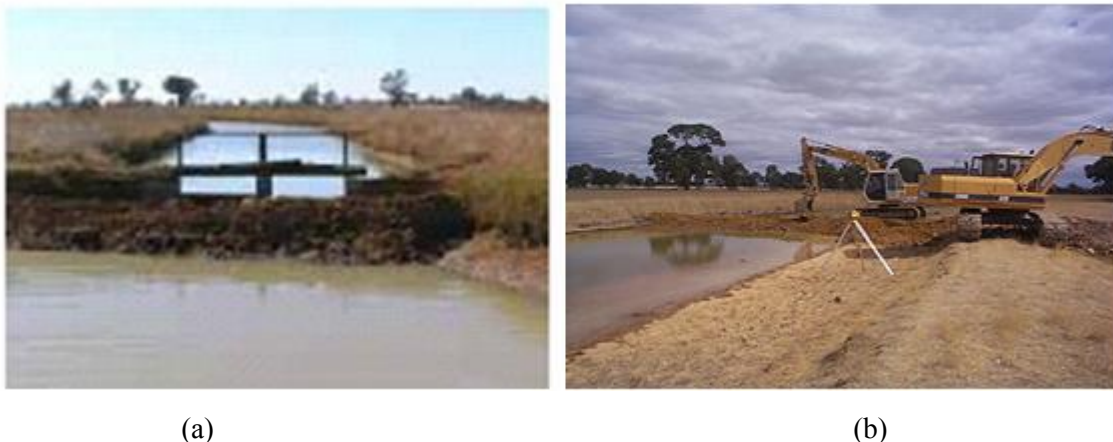
Figure 5: Pondage test for measuring water losses: (a) channel is blocked on both ends, and (b) construction of embankment in progress
